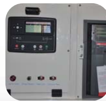
Control Panel & MCB
